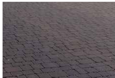
Highway - Tumbled concrete paviours
